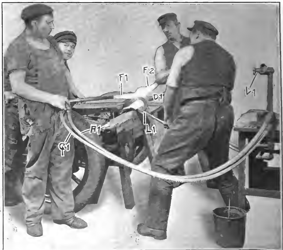
Fig. 2—Straightening bent dumb iron of frame by blast heating and using bending iron
